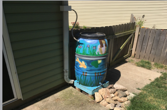
Figure 3. Rain barrel connected to a residential gutter system (credit: Ethan Chitty)
