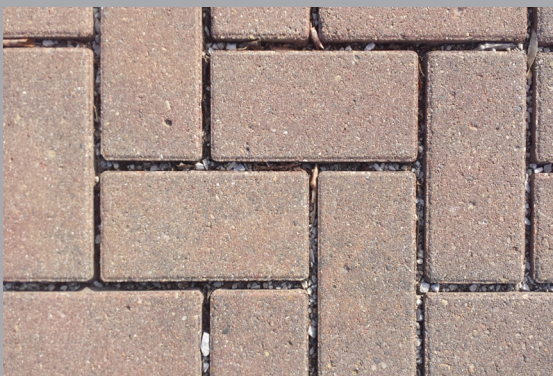
Figure 2. Permeable pavement (credit: Purdue University College of Agriculture)
