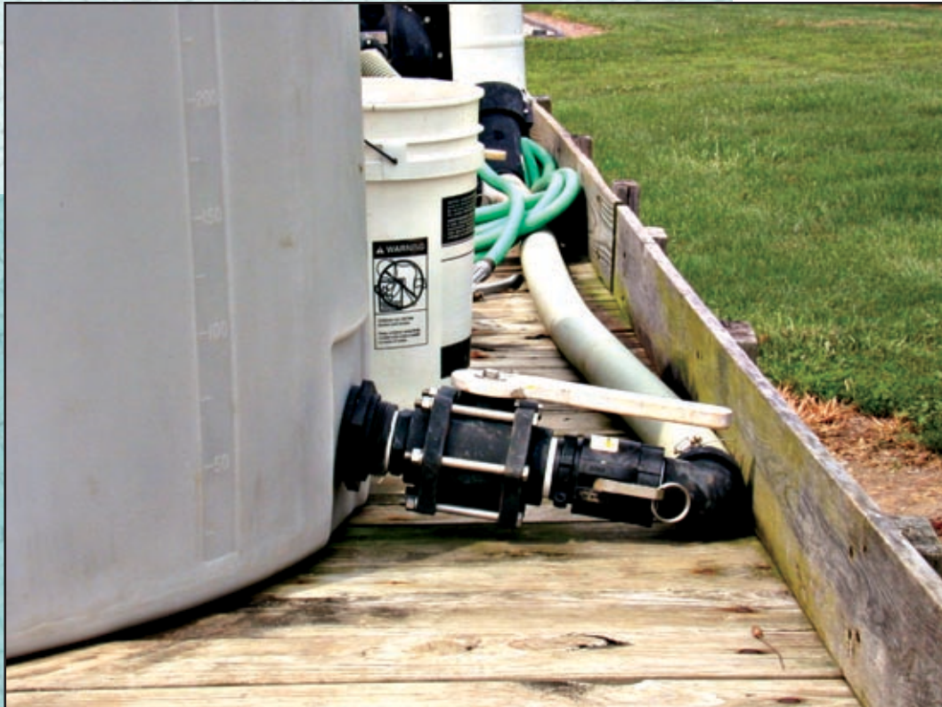
A block is needed to support the valve on this tank.
