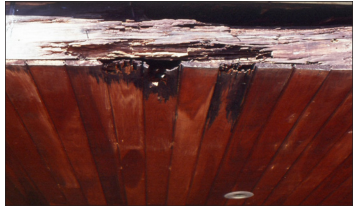
Figure 12. The decayed board ends are cypress sapwood while the sound end is heartwood. The joist is southern yellow pine sapwood.
